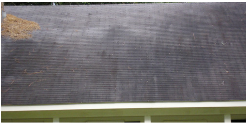
Black stains on an asphalt roof caused by algae.
