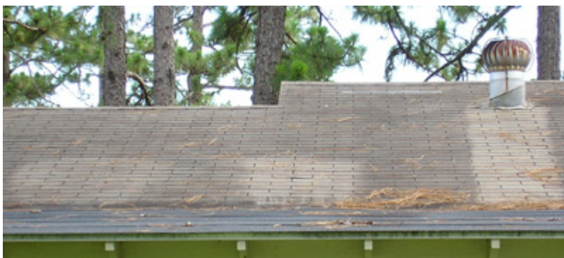
Roof cleaned with oxygen bleach (left) and chlorine bleach (center). Galvanized vent (right) prevented algae growth.
