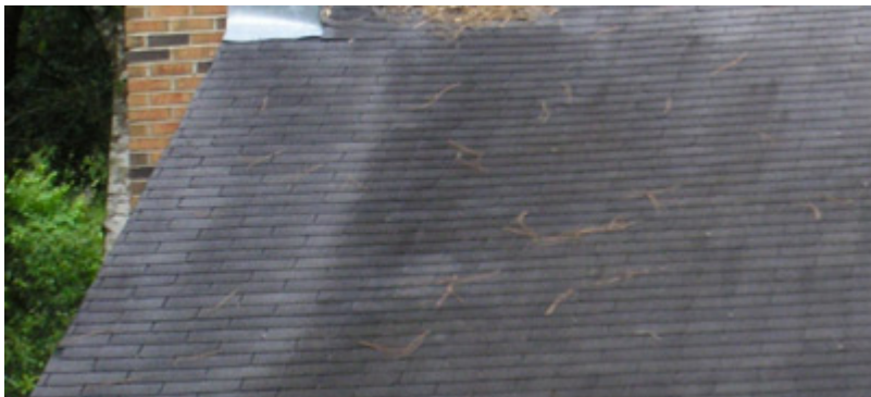
Absence of algae under metal flashing
